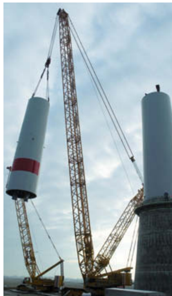
Setting up a tower section of the 115 meters high steel tube tower on the DEWI OCC test field in Cuxhaven. Photo Jens Hadel
