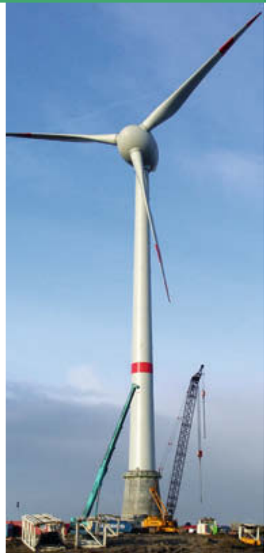
The eighth E-112 wind turbine is completely assembled and could be put into operation as planned by the end of 2005. Photo Jens Hadel
