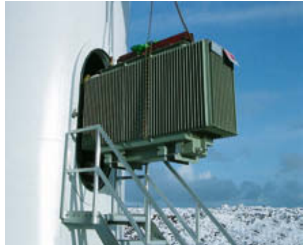
Both transformers and towers were designed to accelerate any necessary transformer replacements. Transformers can easily be replaced within just a few hours.
